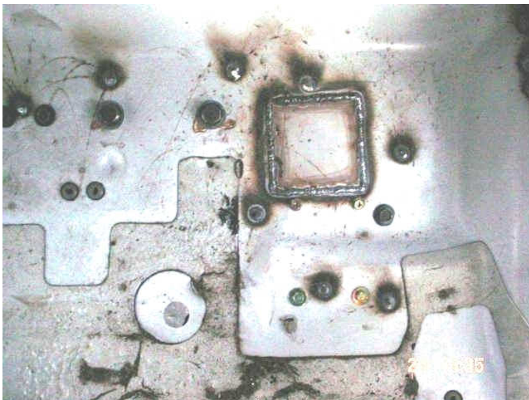
An example of a patch-weld in the central floor area of another vehicle, ready to clean up and coat with automotive epoxy primer.
