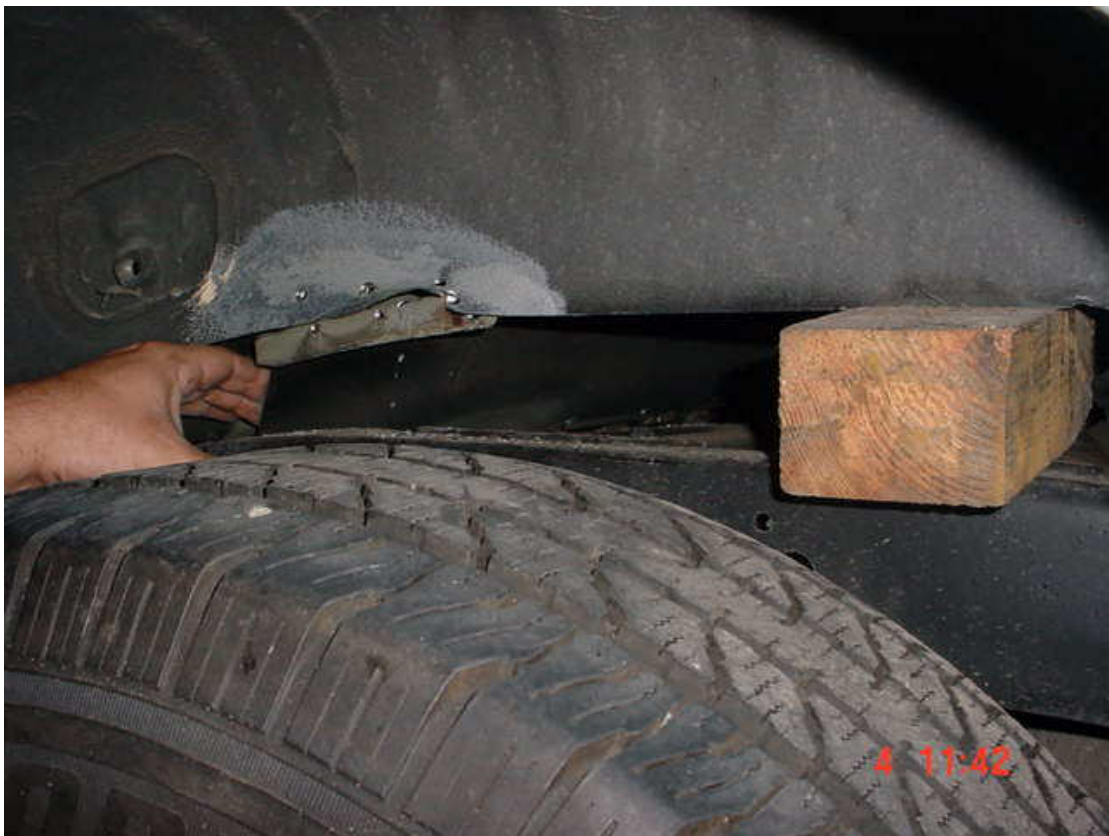
After drilling out the 4 wheel-arch spot-welds, a check is made by levering to ensure that all other spot-welds have been drilled out, to allow reinforcing plate to be easily removed.
