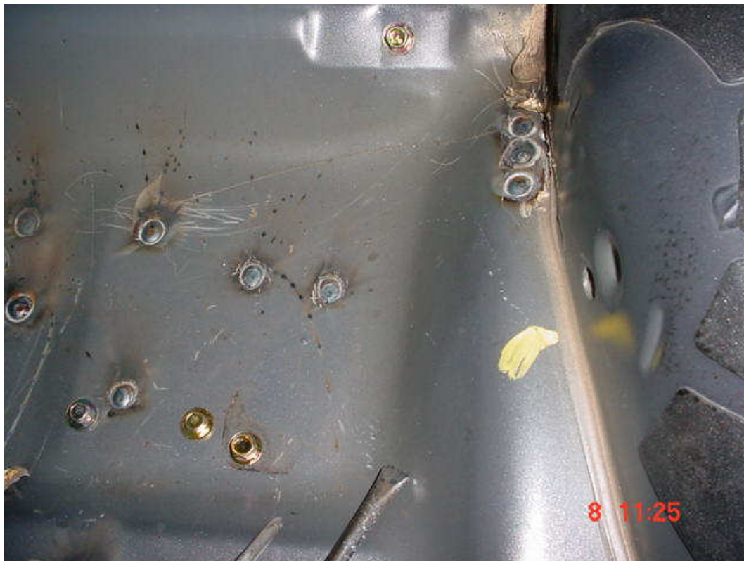
Plug-welds in the central floor area have been welded, ready to grind flush.
