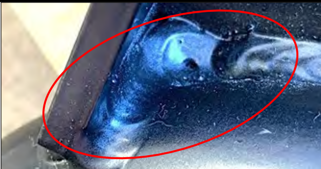
Image 5: This is an example of an incomplete weld and craters, at the ball joint end housing (a highly loaded part of the arm).
